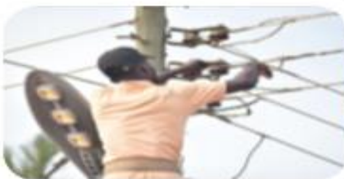
Provision of 500 Streetlights at Akropong, Amanokrom, Mamfe, Okorase, Osebene and Larteh
